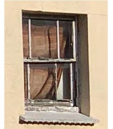
Cross Street- rotten, double glazed required
