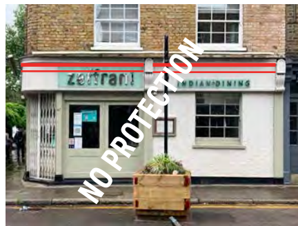
47 Cross Street, Fascia sign too large bad flashing, Cornice
