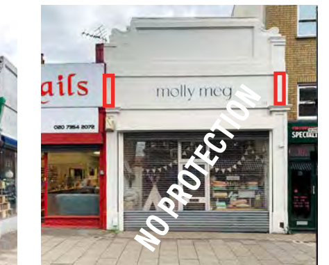
111 Essex Rd, Brackets missing external shutter, door location
