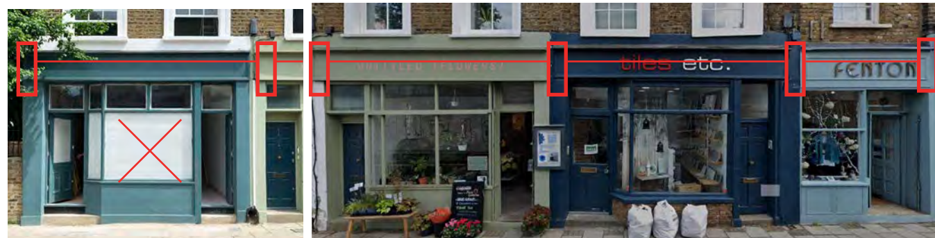
8, 6, 4 and 2 Shillingford Street, Heritage damage allowed to continue no Console Brackets or Cornice.
