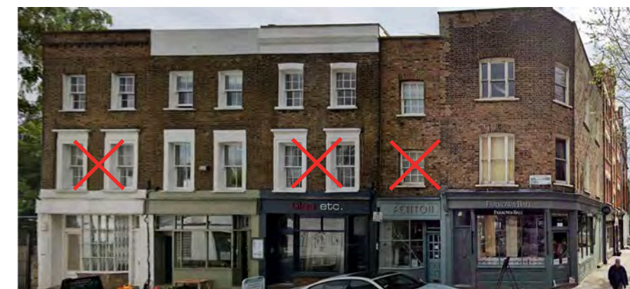
8, 6, 4, 2 Shillingford Street, 38 Cross Street. Victorian windows have been fake georgianised. All replaced with 1 over 1 triple glazed.
