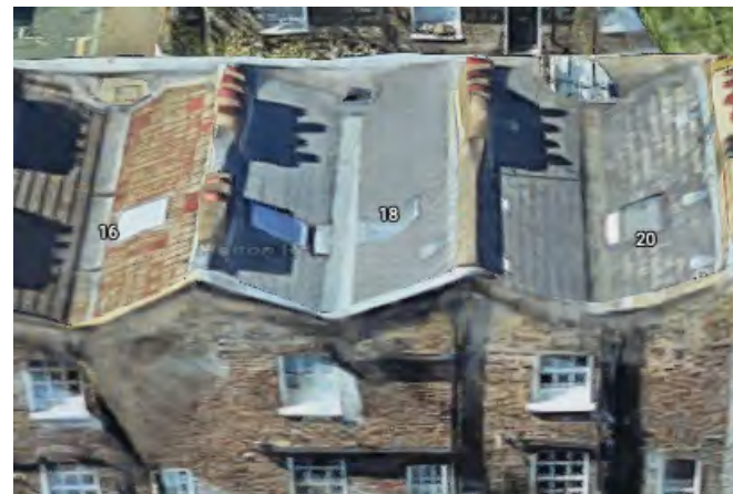
Inverted Pitch roof known as London or Butterfly roof. With V Parapet rear.
