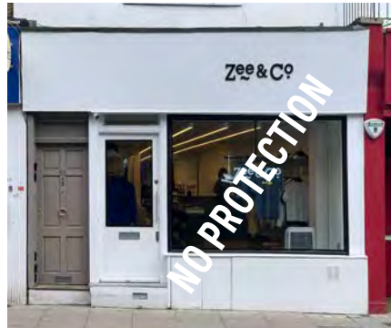
58 Cross St, Fascia Oversize missing Cornice and Brackets
