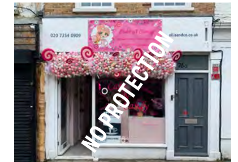
76 Essex Road, sign obstructs cornice and fascia
