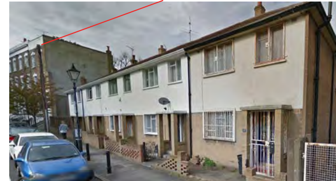
2, 3, 4, 5, 6 Dagmar Terrace /rear garages Lost heritage 4 storey terrace infill with out of scale 2 storey modern terrace damaging the Conservation Area. Poor windows and details suitable for external insulation, new windows, and additional storeys.
