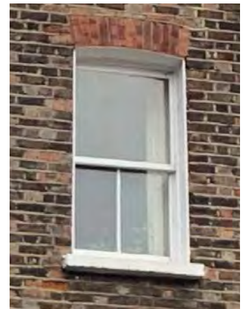
Cross Street- Harmed sash on listed Georgian
