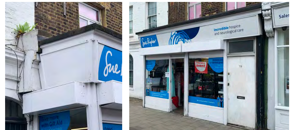
72 Essex Road, shop extension built tight on centre of party wall (or even over the line) not to inside as normal with shops. Roller shutter box extends in front of neighbours window!!
