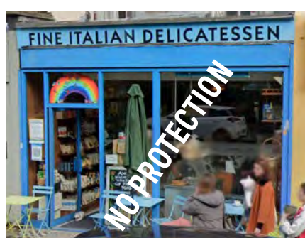
46 Cross St, cornice, brackets Aluminium, needs rebuild
