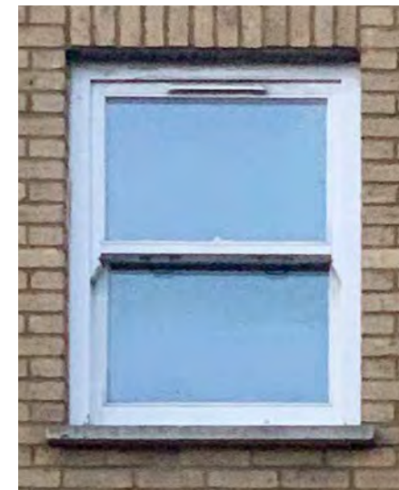
Essex Road, - New build trickle vent slot in top sash
