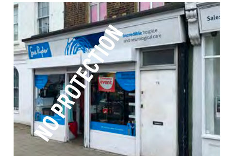
72 Essex Road, roller shutters sign obstructs cornice fascia
