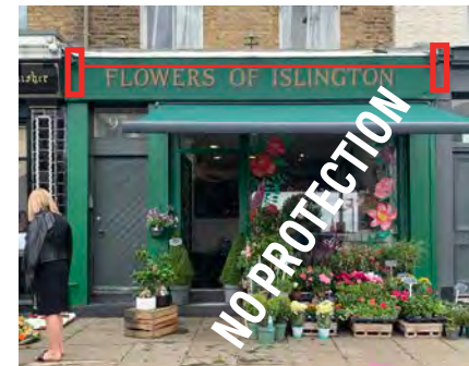
97 Essex Rd, Cornice and Brackets missing
