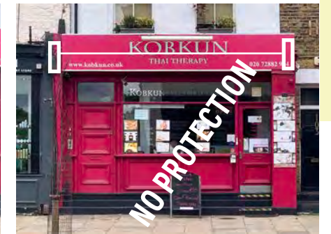
101 Essex Rd, Cornice and Brackets missing
