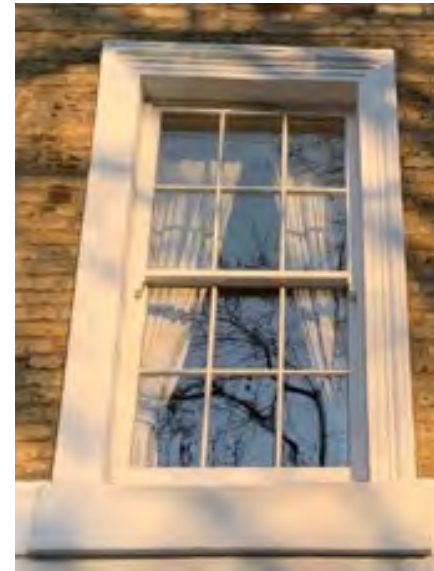
Timber double glazed example with no secondary reflection. This is from an Islington CA.
