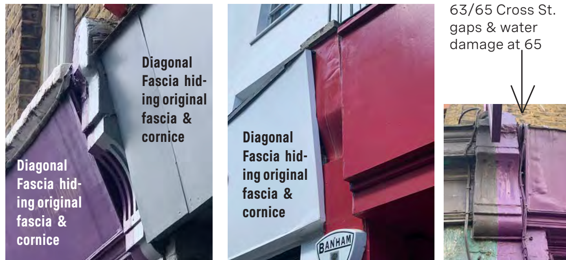
65/67 Cross Street, Signage Fascia large, obstructs bracket
