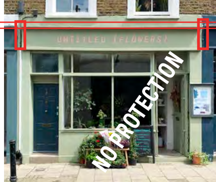
6 Shillingford Rd, Cornice and Brackets missing
