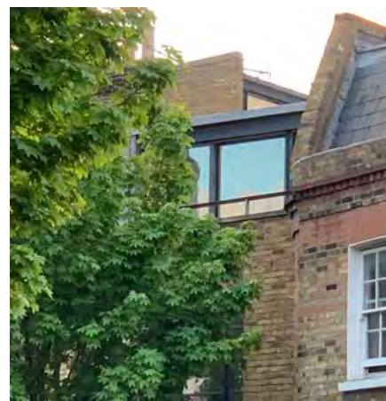
64 Cross Street modern exemplar discussed in 2006 Design Guidance. Slim roof with large south glass and no brise soleil. Overheating.
