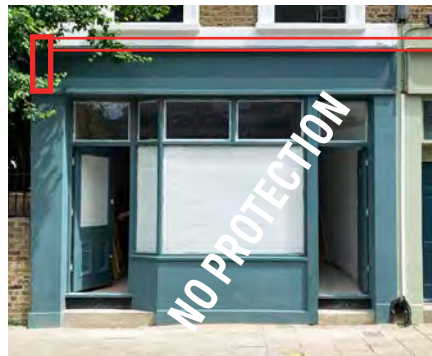
8 Shillingford Rd, Cornice and Brackets missing
