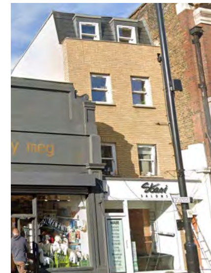
113 Essex Road Modern interpretation lacking historic details suitable for external insulation.
