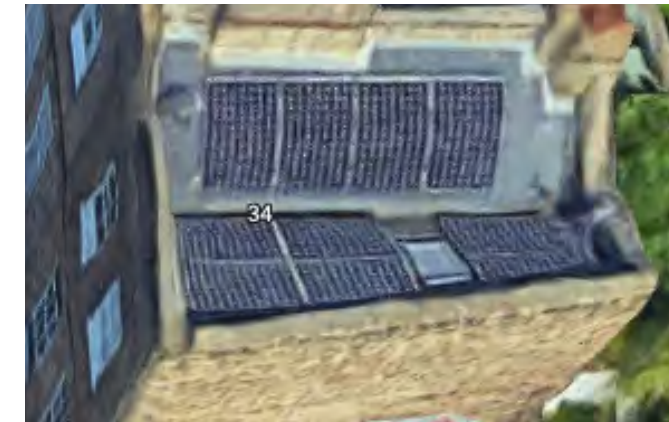
34 Halton Road hidden system, 10 panels
