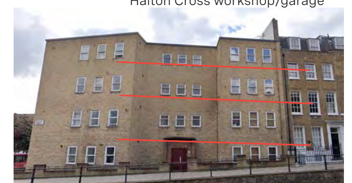
1-8 Belmont House, Cross Street Poor windows, details, and facade composition out of alignment with Heritage Terrace . Suitable for external insulation, and facade details.
