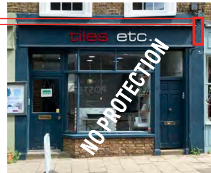
4 Shillingford Rd, Cornice and Brackets missing
