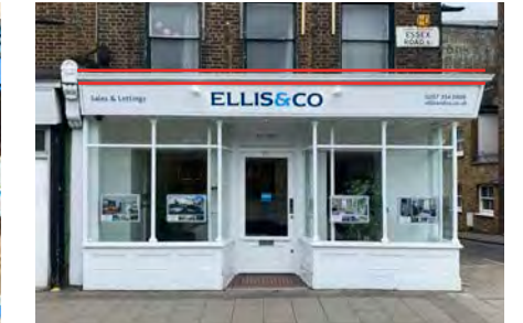
70 Essex Rd, Cornice missing
