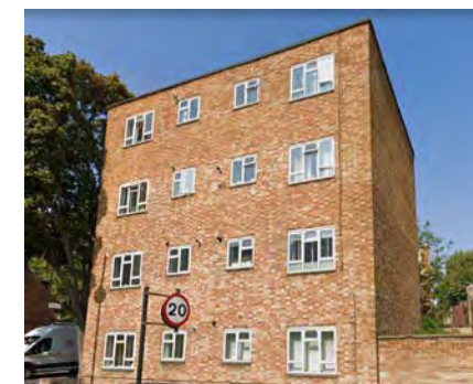
9-16 Fircroft House, Halton Road Poor finishes, PVC windows, and out of scale, suitable for external insulation, new windows, and balcony/ facade extension.
