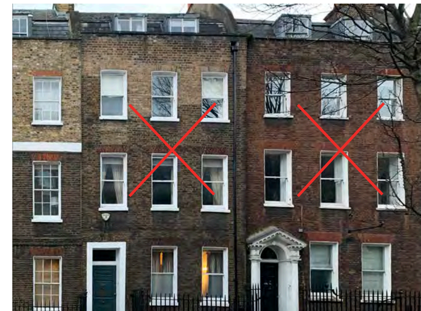
Harmed 1 over 1 windows should be replaced with sympathetic historic pattern 6 over 6 double glazed, Cross Street Listed terrace
