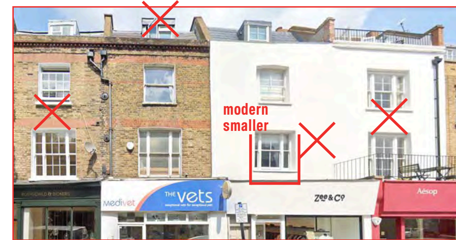
62 (fake georgianised), 60, 58 (modern smaller), 56 Cross Street. All dormers wrong. Suitable 1 over 1 simulated sash triple glazed
