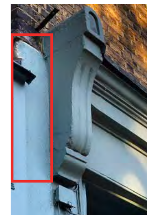
38 Cross Street, left missing Console Bracket
