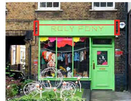
41 Cross Street, Cornice and Brackets missing
