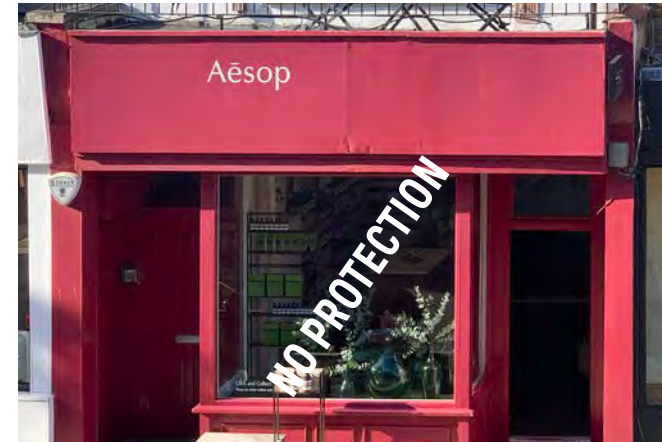
56 Cross Street, Damaged Console Bracket, No Cornice, Signage Fascia too large, Out of Scale.
