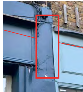
4/2 Shillingford St, missing Console Bracket
