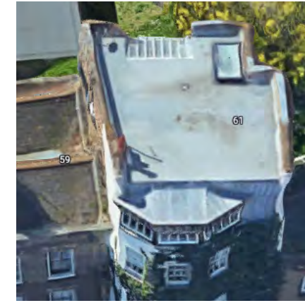
Modern Membrane Flat roof, new floor added to a Listed Building. 61 Cross St
