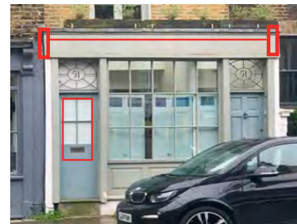
51 Cross Street, Now a House, Cornice and Brackets missing
