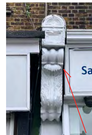
70 Essex Rd, bad gaps
