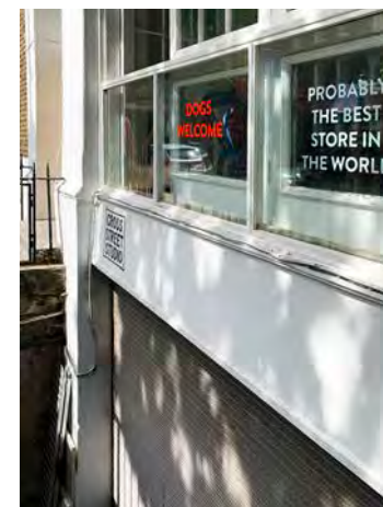
26 Cross St, Harmed Roller Shutter basement
